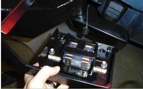
Figure 14: Blind Spot Sensor Installation
