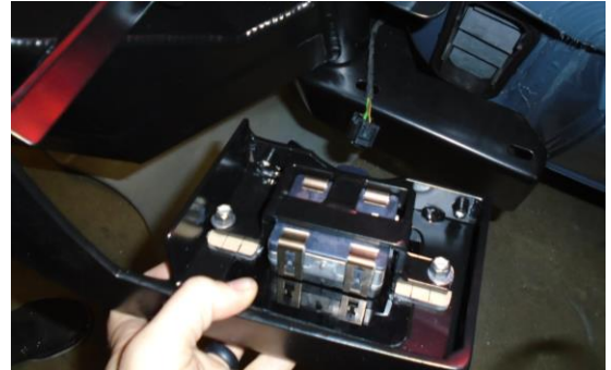
Figure 14: Blind Spot Sensor Installation
