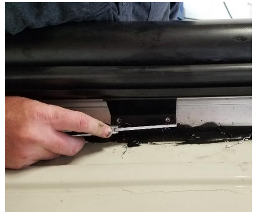
Figure 7. Drill out rivets and cut sealant around awning brackets to unmount one side of your roof rack.
