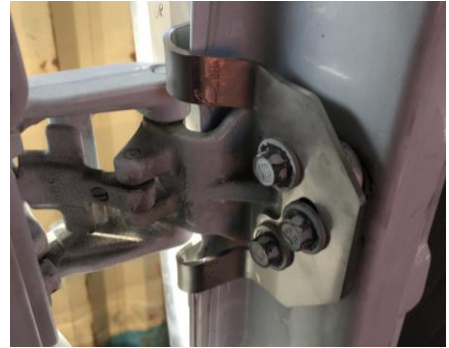
Figure 5: Inside View of Installed Upper Hinge
