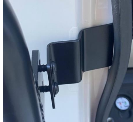
Figure 16: Example of gap between bracket and rack
