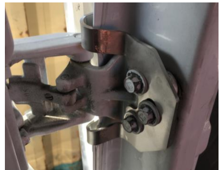
Figure 5: Inside View of Installed Upper Hinge
